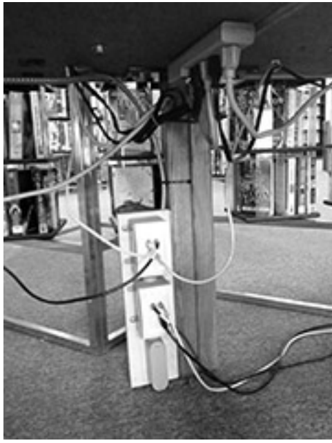
Inadequate wiring and lack of plug-ins for electronics in the present library. Courtesy Leo A. Daly Co.
