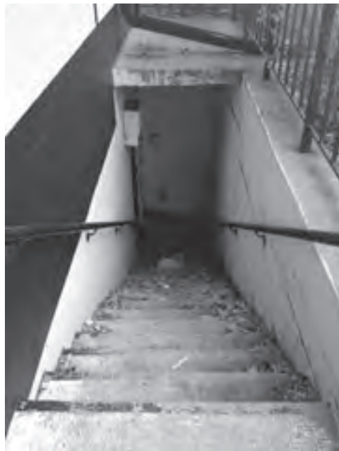
Outside stairwell to the basement level of the present library. Courtesy Leo A. Daly Co.
